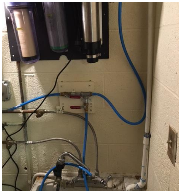
Photo 5: Merlin water purification system, installed at St Luke's Center in Flint, Mich.
