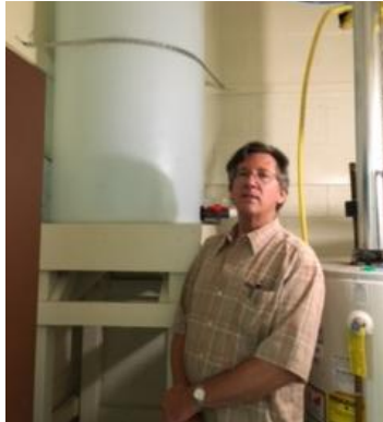
Photo 7: Raised tank of purified water, strapped to the wall. Joe Novitsky, principal engineer in photo.
