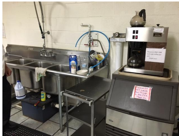
Photo 8: Purified tank water, output into the kitchen through the blue hose. Purified water is directly plumbed into the ice machine – the only automatic ice machine in Flint (ironically in a center for homeless kids).
