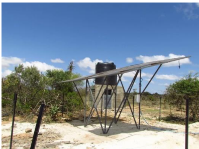
Photo #1: the well set up. Solar panels (since we live many miles off any electrical grid) power a pump, underground pipes with fill that 10k liter tank on top of a building. Gravity fed water outlet on the building, to which the water purifier is attached.
